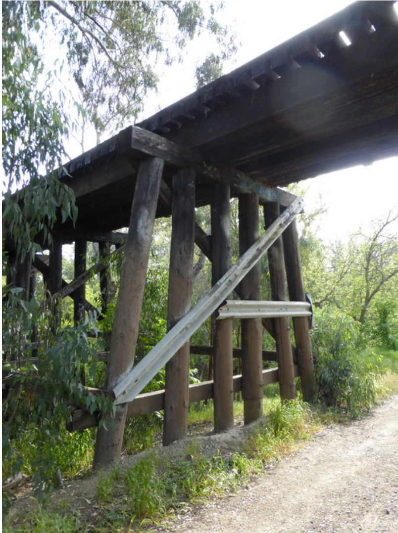
Figure 11. Western Pacific Railroad pile-bent trestle bridge over Coyote Creek, near Story Road, San Jose, one of three extant pile-bent trestle bridges in Santa Clara County.
